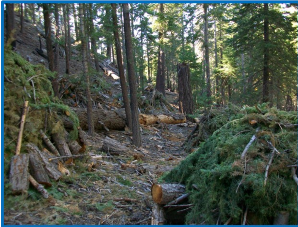
Logan Creek thinning and CWD reduction project on the north aspect of the drainage, October 2011. SNPLMA Round 9 funded. Piles burned November 2011.
