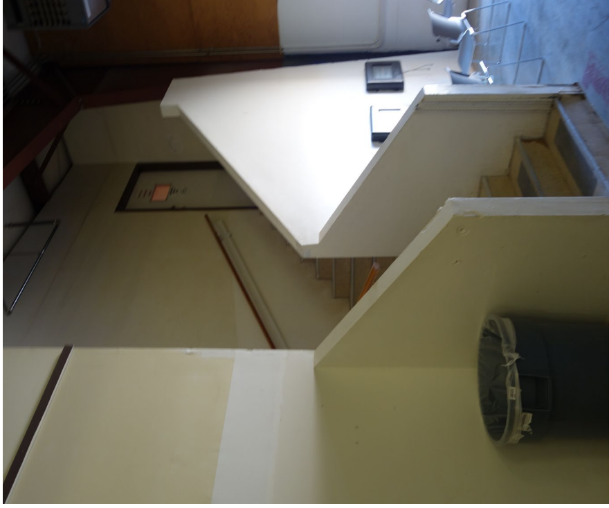
MPR / Visitation / NDF Shop – FCA Building #1898
